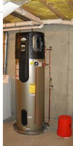
Hot water heater
